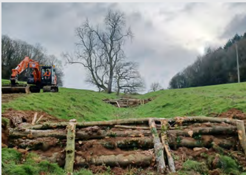
Construction on a leaky dam
